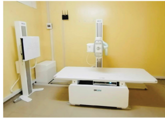
ST. DOMINIC MISSION HOSPITAL NDOLA, DRGEM DIGITAL X-RAY MACHINE INSTALLATION - APRIL, 2023
