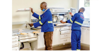
NEW MAINA SOKO MEDICAL CENTRE - LUSAKA. INSTALLATION AND USER TRAINING OF: 1. CARESTREAM CBCT/3D X RAY MACHINE 2. FOUR DENTAL SYSTEMS 3. DENTAL LABORATORY EQUIPMENT 4. CSSD: LARGE AUTOCLAVES, WASHERS-AUGUST 2020
